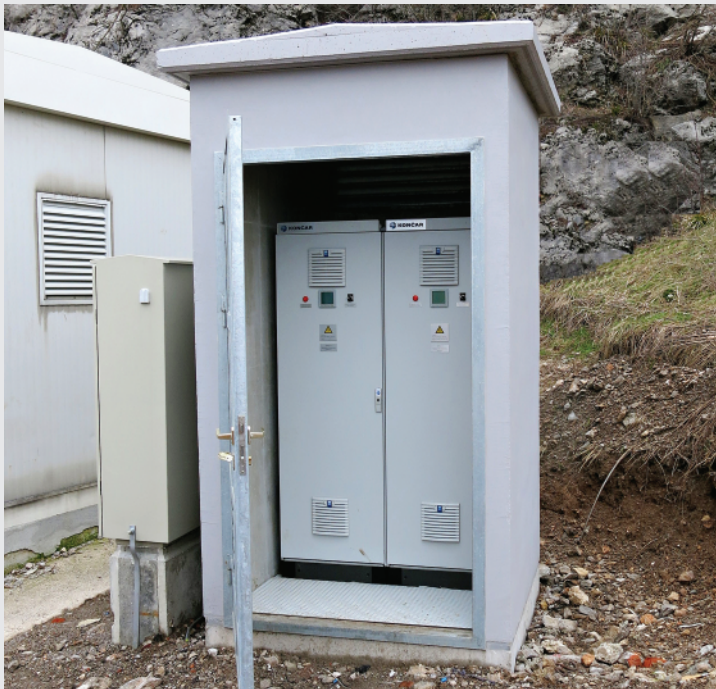
Two converters KONTRAC PN 30 AC installed in Drivenik Railway Station, Croatia
