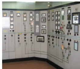
control and signalisation
