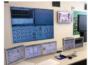
monitoring and emergency lighting
