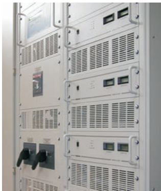
Detail of new systems +24 V
