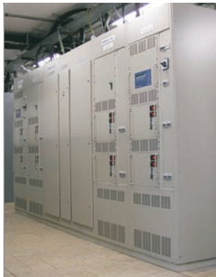
New modular rectifiers 220 VDC in the facility
